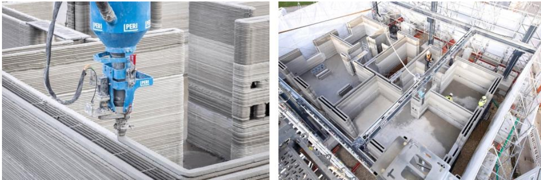
Figure 2.9 Left: 3D printed concrete filaments. Right: Top-down view of the construction site (PERI GmbH, 2020)
